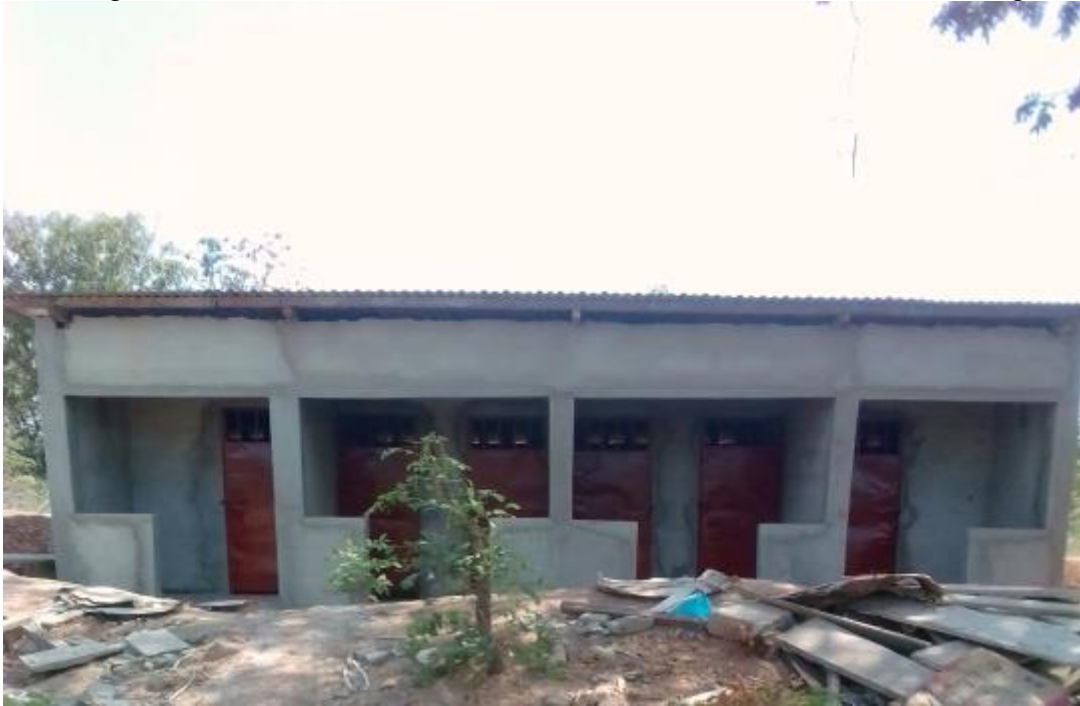
Building with 4 toilets and 2 showers of the medical center SAREPTA of Tangafila
